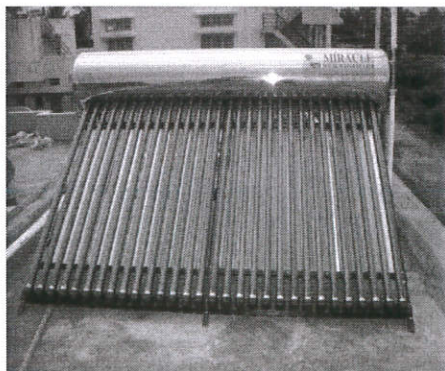
Evacuated Solar Water heater
